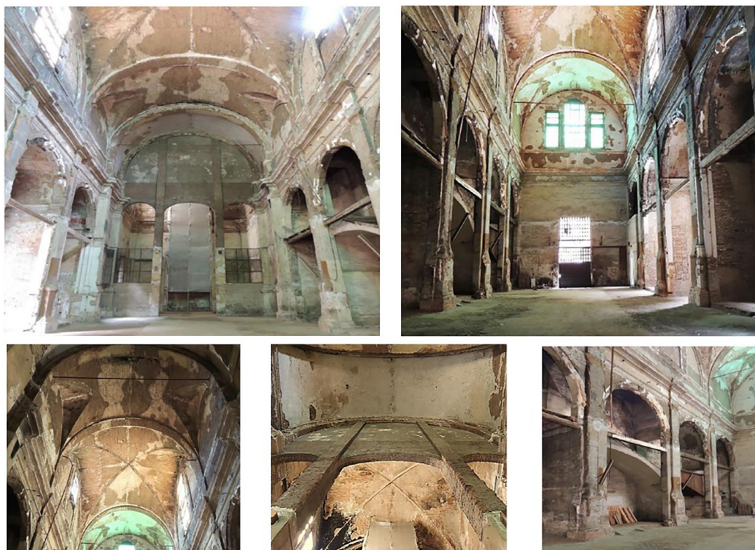
Fig. 4. The bad maintenance conditions of the internal space of the former church. Source: Authors' own photographic report.
