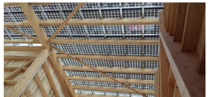
Figure 0-10 Warehouse installation in Switzerland, by Galaxy Energy, 33.41 kW, with
