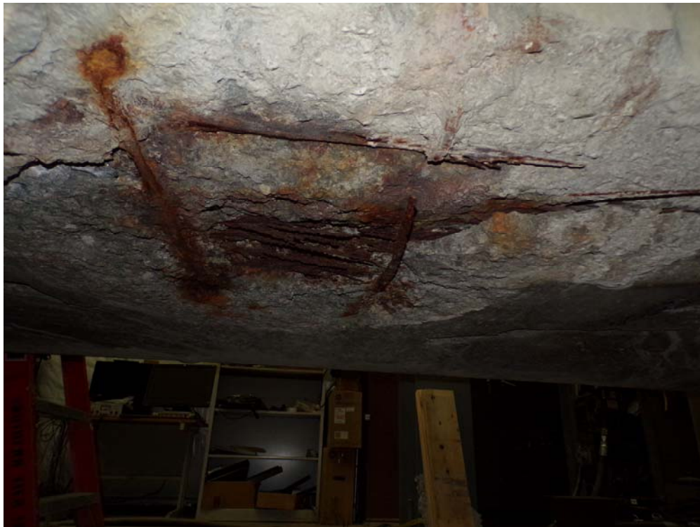
Figure 4.19: Exposed and corroded strand in bottom of Specimen E3
