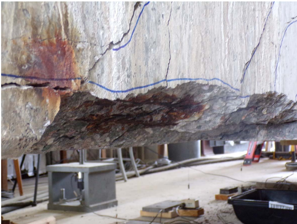
Figure 6.15: Visible strand corrosion and section loss in Specimen E9 after spalling of concrete
