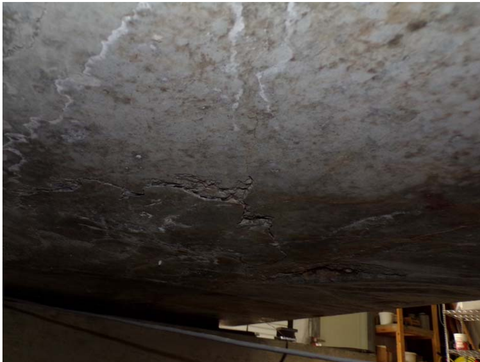
Figure 4.15: Bottom Surface Deterioration (Specimen E4)
