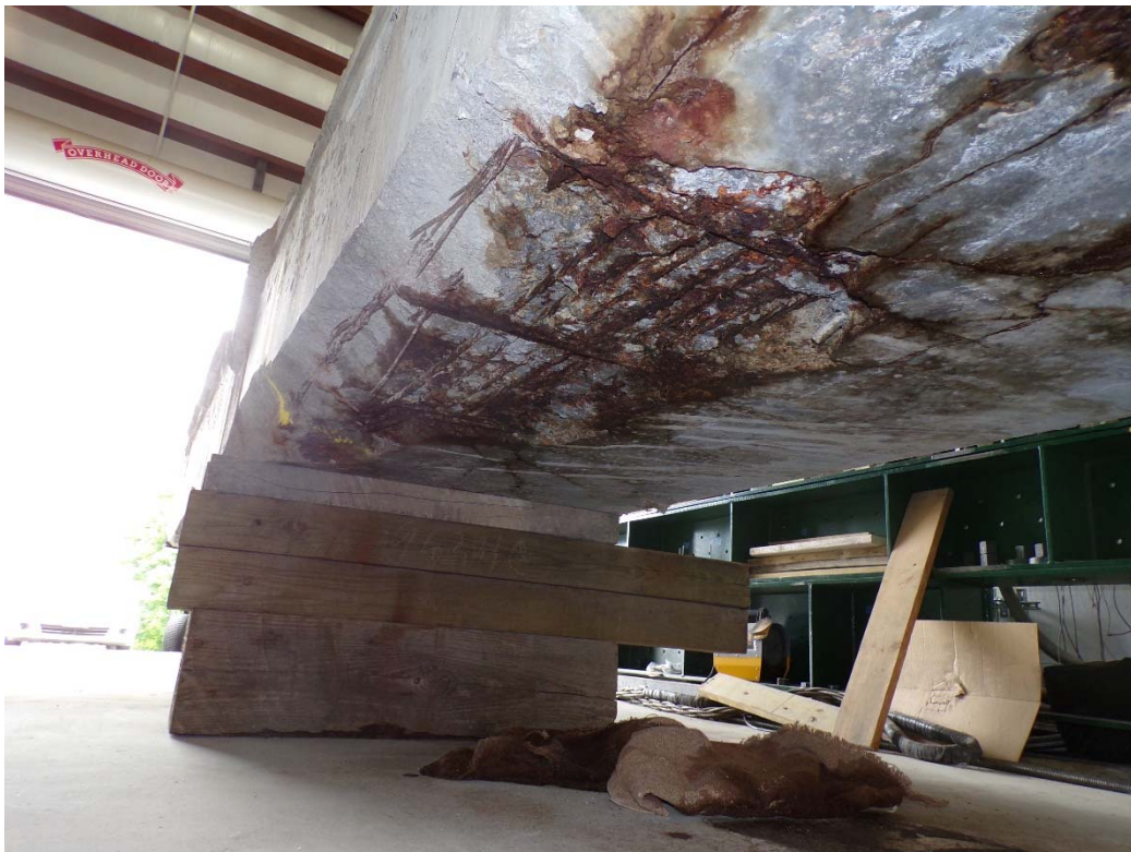
Figure 6.12: Specimen E3 showing visible deterioration of strands after spalling of concrete cover
