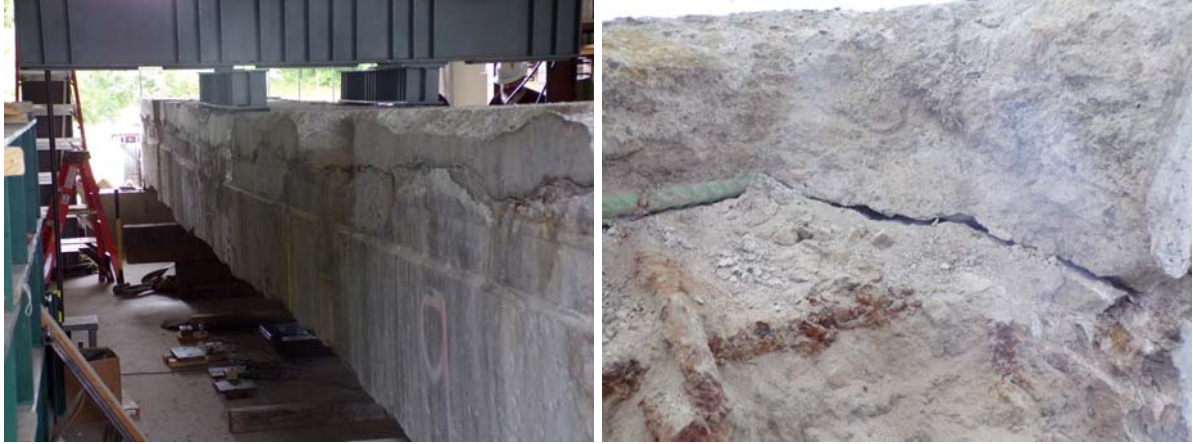
Figure 5.30: Debonding of concrete overlay in Specimen E9 (north shear span)
