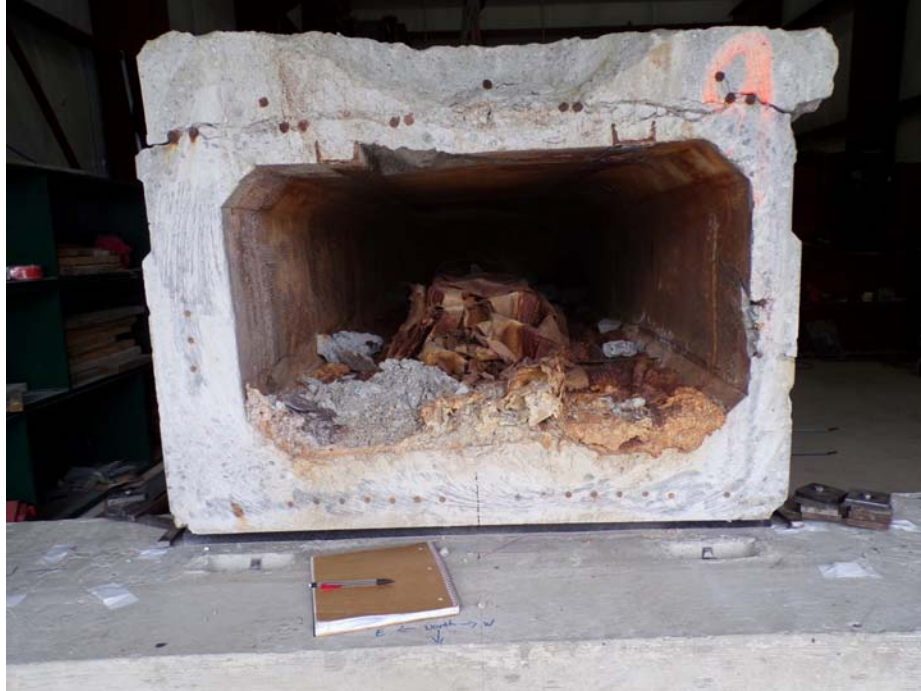
Figure 4.24: North end of Specimen E9
