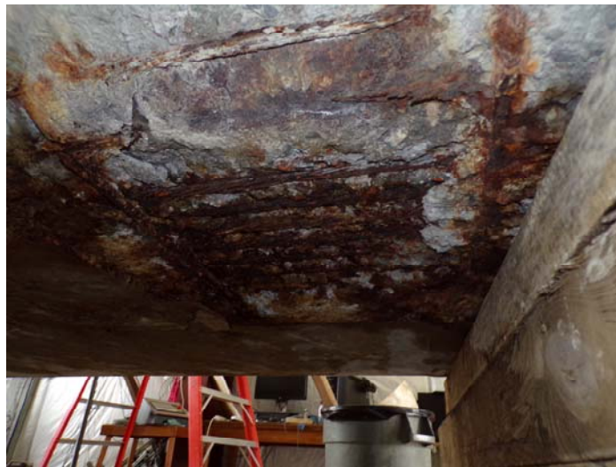
(b) View of Section 3 after the test
