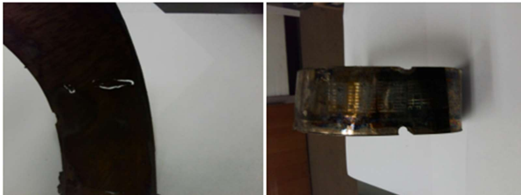
Figure 49: The flaws after removing the PET base with heat treatment.
