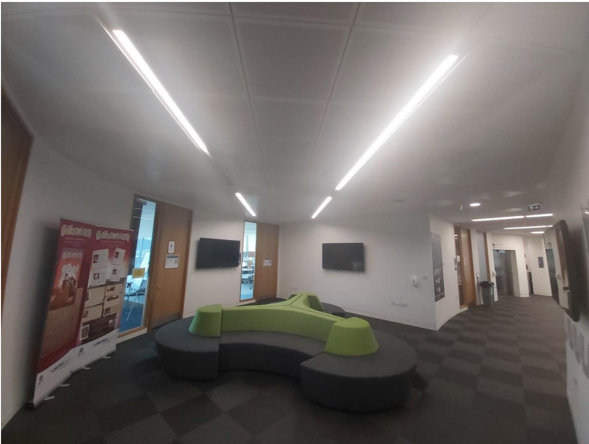
Figure 5.7: Waiting Space at the Classroom area with a Surface IP66 Led Dimmable Linear Luminaire lighting fixtures (Oastler Building).
