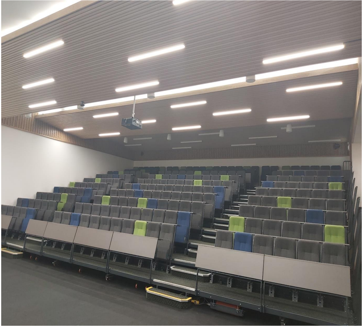
Figure 5.3: 300-Seater Lecture Theatre with the Surface IP66 Led Dali Dimmable Linear Luminaire Lighting Fixtures and Central Heating System (Oastler Building).
