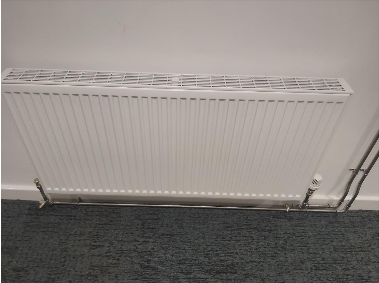
Figure 5.13: Surface Heating System (Percy Shaw House Building).
