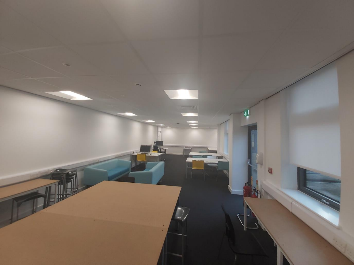
Figure 5.10: Post Graduate Room Recessed Led 600 x 600 Dali Dimmable LG7 Luminaire C/W Ribbed Polycarbonate Refractor Lighting Fixtures furnished with Central Heating Fixtures (Percy Shaw House Building)
