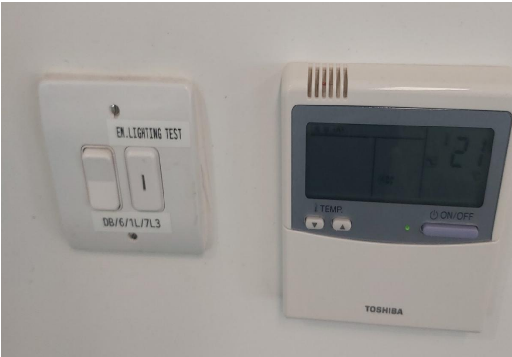
Figure 5.4: Controls for the Lighting and Heating System (Oastler Building)
