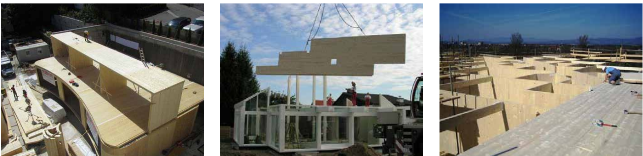
FIG. 3.3 From the left: Prefabricated CLT elements are transported to the construction site and then assembled and erected manually – Waldorf School in Ljubljana, Slovenia.
