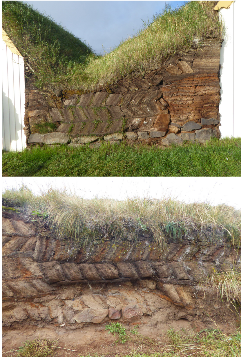
Figure 2: Replacement of individual turf blocks as ad hoc, in situ replacements, Skagafjörður area, Iceland. Top: main farm buildings at Glaumbær Museum; bottom: multi-phased wall repairs of an outbuilding at Tyrfyngsstaðir. Photographs: Tanja Romankiewicz.
