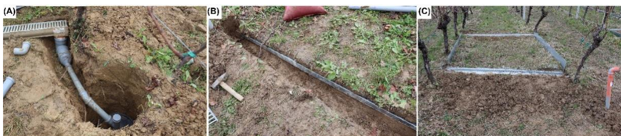
Figure 4. Process of installation of surface runoff collection instruments: (A) collection tank placement and pipe connection, (B) flow guide placement (C) border and drain channel placement at the SUPREHILL Critical Zone Observatory (CZO).
