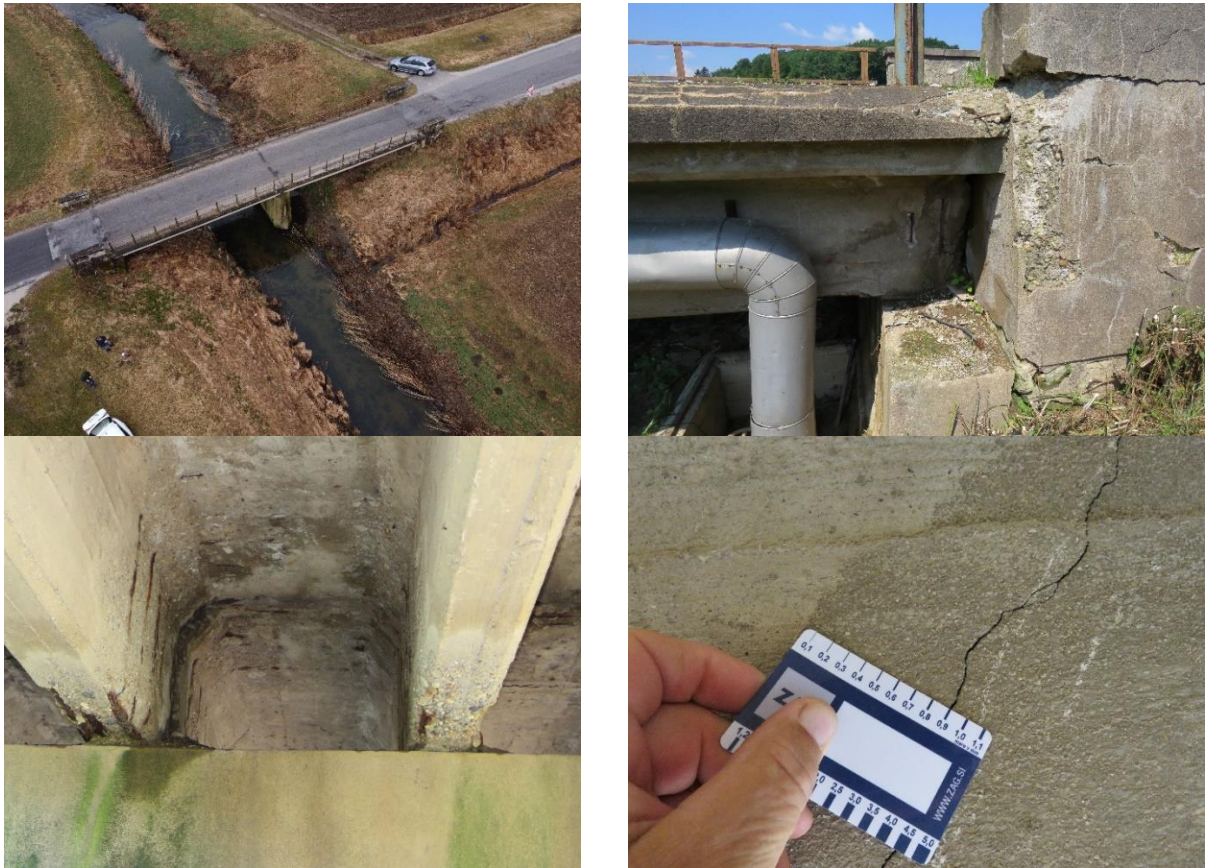
Fig. 2: Location of bridge (upper left), abutment with bearing of end girder (upper right), deterioration of concrete and steel corrosion (down left), shear cracks 0.9 m wide (down right).
