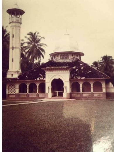
Figure 9. The New Great Mosque of Rantauprapat under construction (Source: Personal Document of the BKM Masjid Agung Rantauprapat)
