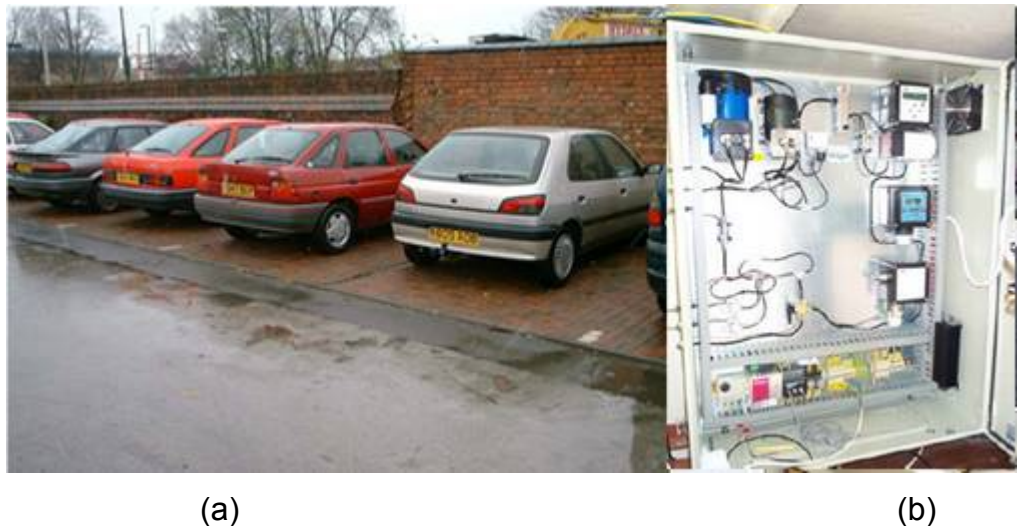
Figure 1: (a) Part of the experimental pervious car park (consisting of pervious block paved and porous asphalt surfaces and both stone and plastic box storage elements) constructed under the candidate's direction in Coventry (from Newman, 2004b) and (b) the gas monitoring system (photograph by Tim Puehmeier).
