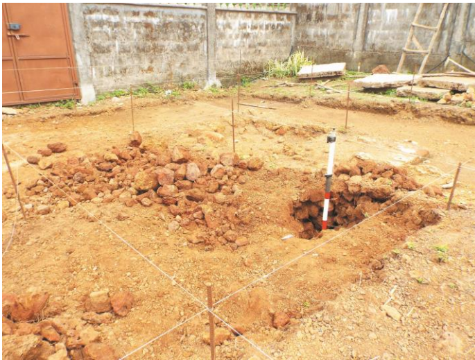
Figure 4.7a: The testing of a section of the interior of the house. (Source: Photograph by the Author)
