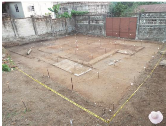
Figure 4.5b: Excavation of the house area after completing Level 1. (Source: Photograph by the Author)
