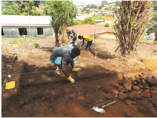
Figure 4.22a: The initial testing of Unit 001 revealing edges of a stone wall and staircase. (Source: Photograph taken by the Author)
