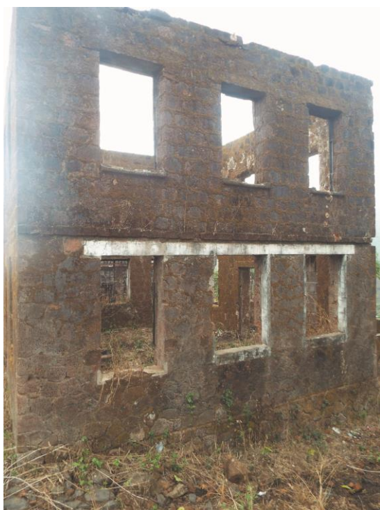
Figure 3.4a: An abandoned stone house located at Dadley Street (circa February 2020). (Source: Courtesy of Érika Melek Delgado)
