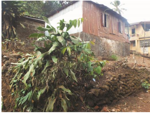
Figure 3.5a: A modified frame house, renovated using corrugated iron roofing sheets, situated along Fitzjames Street. (Source: Photograph by the Author)
