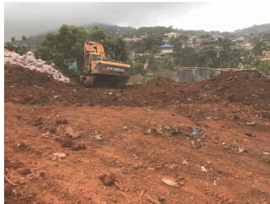
Figure 3.2b: Road construction activities severely impacted the mound representing the remains of a collapsed structure in Locus 21. (Source: Photograph by the Author)
