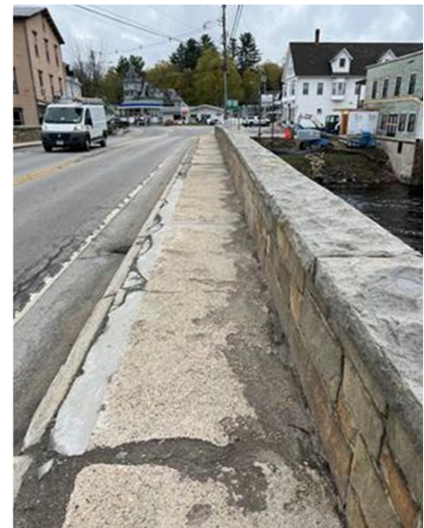
Crumbling and uneven bridge sidewalk
