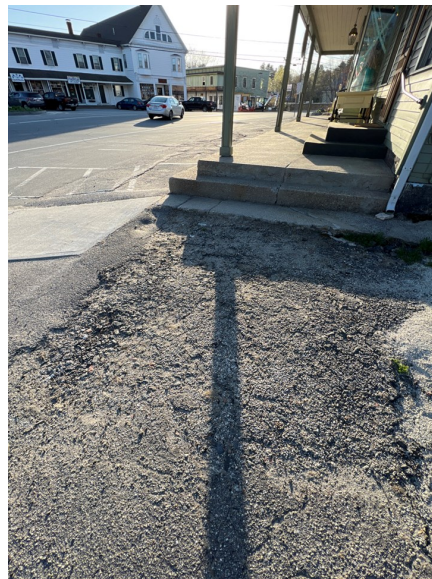
Crumbling sidewalk intersected by steps
