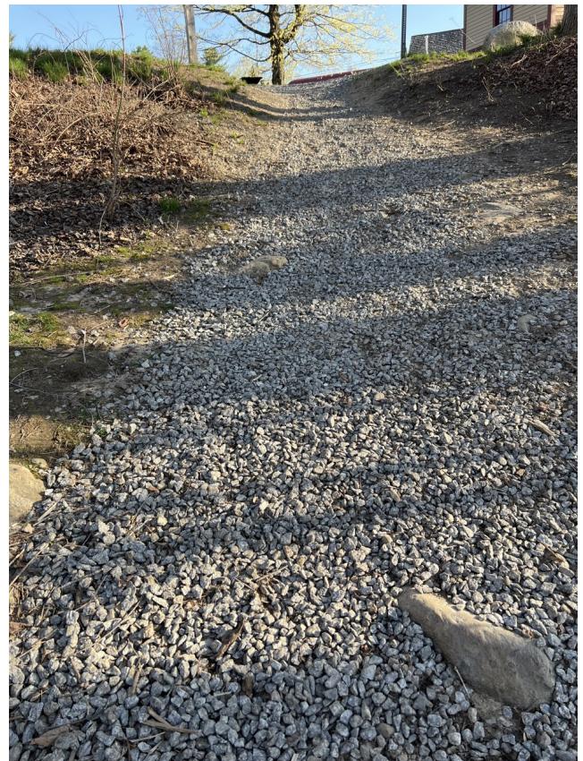
Unstable crushed stone surface of Boat Launch
