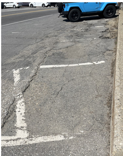
Poorly marked parking spaces
