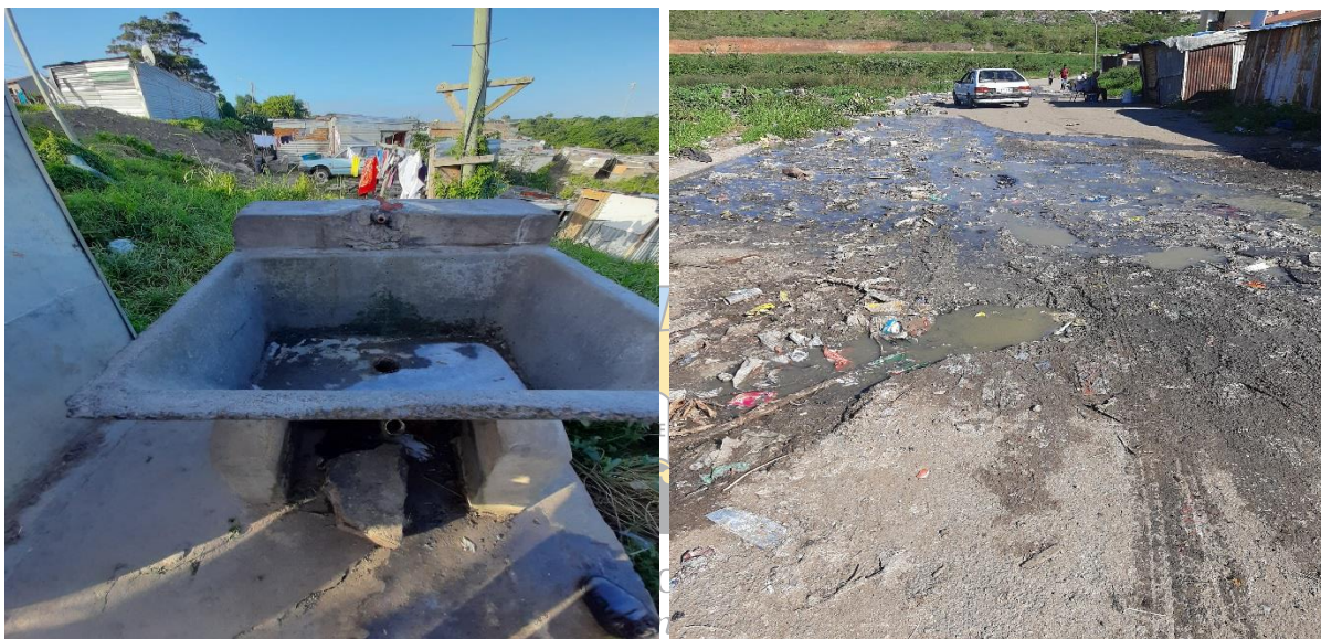
Figure 31a & b: Showing examples of water losses caused by vandalism and theft, and toilet clogs and sewage spillages in ward 6, Duncan Village. Source: (Author, November 2021)
