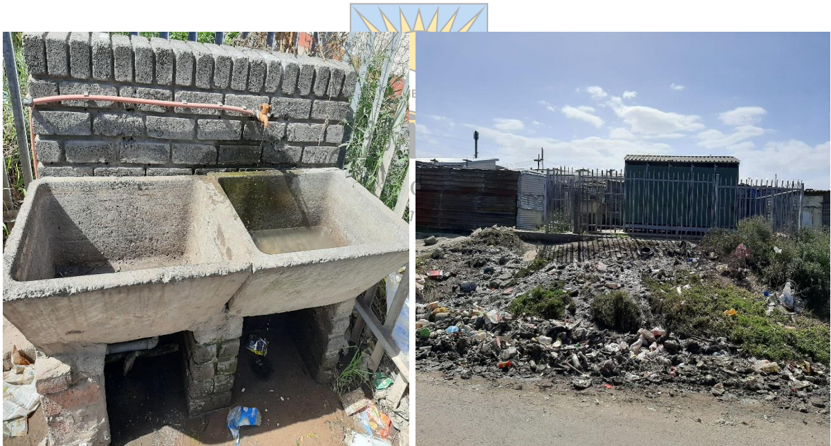
Figure 30a & b: Showing examples of water losses and sewer spillages in Ward 2, Duncan Village. Source: (Author, November 2021)
