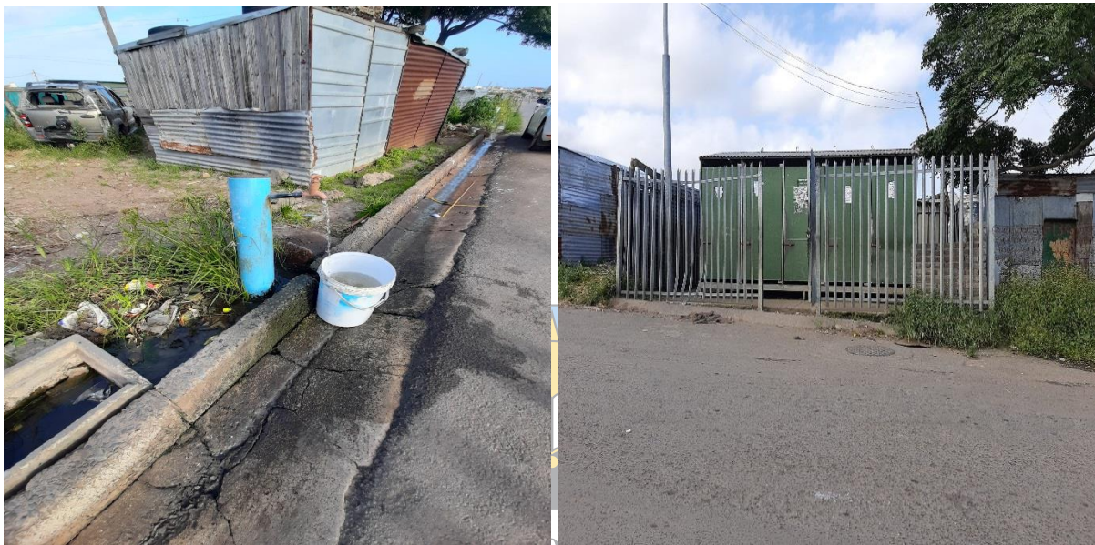
Figure 22a & b: Showing examples of standpipes and communal ablution facilities in ward 1, Duncan Village. Source: (Author, November 2021)
