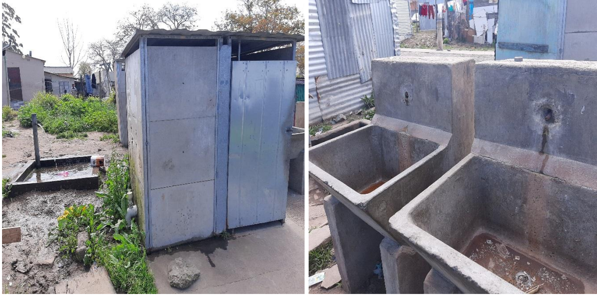
Figure 33a & b: Showing examples of vandalised facilities in ward 8, Duncan Village.
