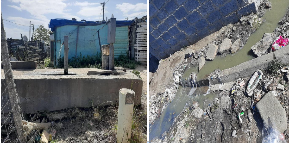
Figure 32a & b: Showing examples of water losses caused by vandalism and theft, and toilet clogs and sewage spillages in Ward 7, Duncan Village. Source: (Author, November 2021)
