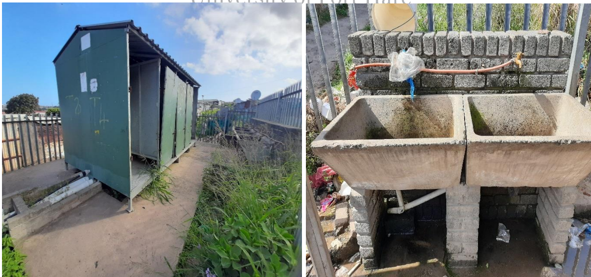
Figure 29a & b: Showing examples of vandalism and theft and poorly maintained water and sanitation facilities in Ward 1, Duncan Village. Source: (Author, November 2021)
