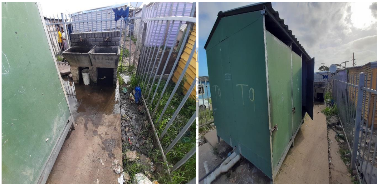
Figure 23a & b: Showing examples of communal water taps in Ward 2 and communal ablution facilities in Ward 2, Duncan Village. Source: (Author, November 2021)
