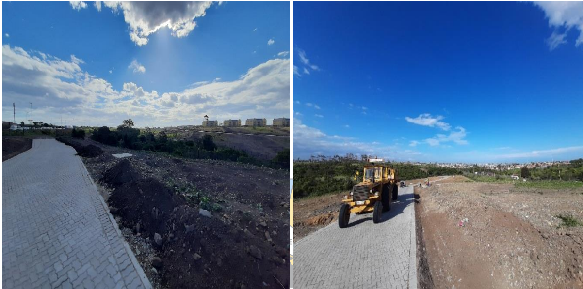
Figure 6a & b: Showing temporary homes sites for Duncan Village informal homeowners in Braelyn. Source: Author (October, 2021)
