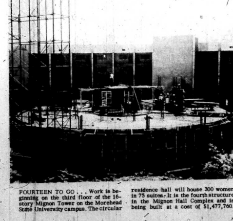
FOURTEEN TO GO . . . Work is being completed on the third floor of the 16-story Mignon Tower on the Morehead State University campus. The circular residence hall will house 300 women in 75 suites. It is the fourth structure in the Mignon Hall Complex and is being built at a cost of $1,477,760.
