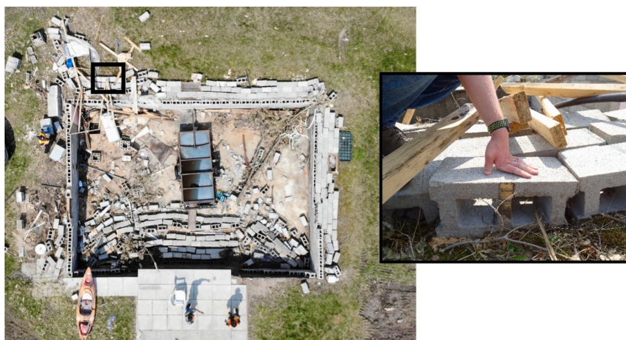
Fig. 7. Drone image showing collapsed basement walls from cottage at Site 6. Inset shows location where floor joists from cottage sat atop of the concrete block basement walls.
