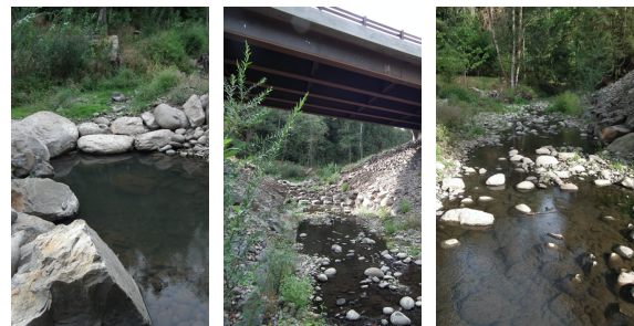
Figures 4A, 4B and 4C. Three different vantage points of Site I.
