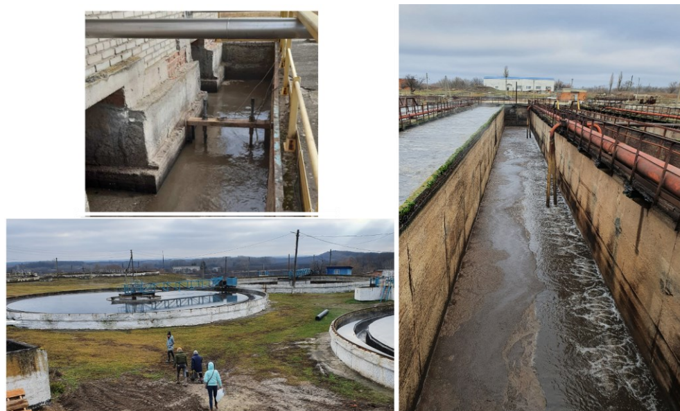
Figure 4. Local WWTP (2021): the measuring instruments are installed at the head of the operating system after the mechanical grids.
