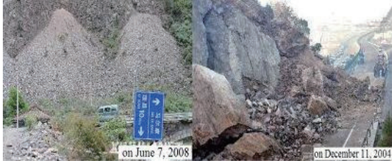
Fig. 1. Disruption traffic for Collapse
