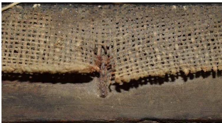
Figure 2.10: Corroded bent nail shaft causing oxidation and loss in the canvas.
