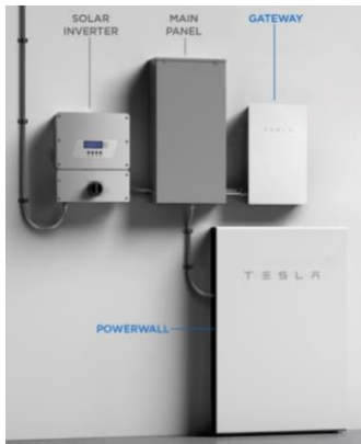
Exhibit 6: Tesla Powerwall System Setup
