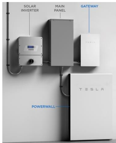
Exhibit 19: Tesla Powerwall System Setup
