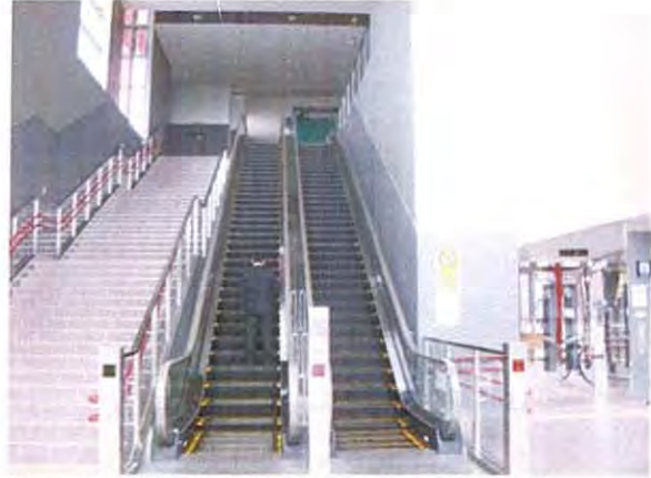
Photo 2. Lift(Right) and Escalator(Center) of West Exit
