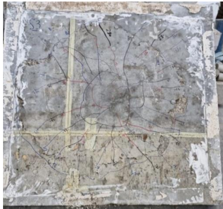
(c) Crack patterns of S3
