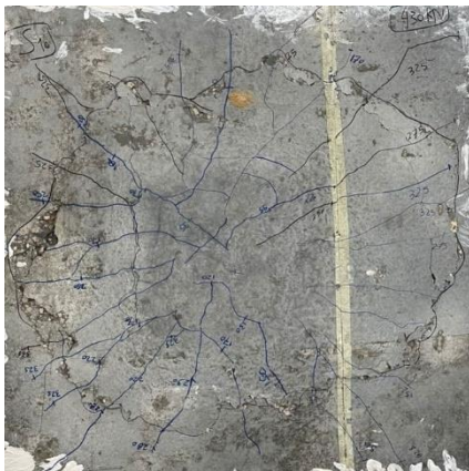
(j) Crack patterns of S10
