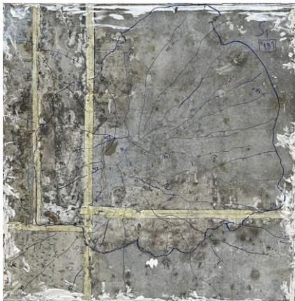
(i) Crack patterns of S9
