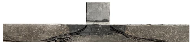
(c) Crack patterns of S3
