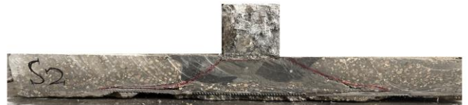
(b) Crack patterns of S2
