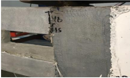
Figure 14. Debonding of the GFRP sheets
