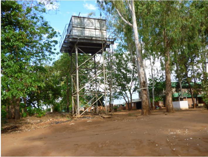
Plate 6.2: A borehole at Neno Health Centre, Malawi, fitted with a motorized pump, supplying water to the facility through an overhead tank
