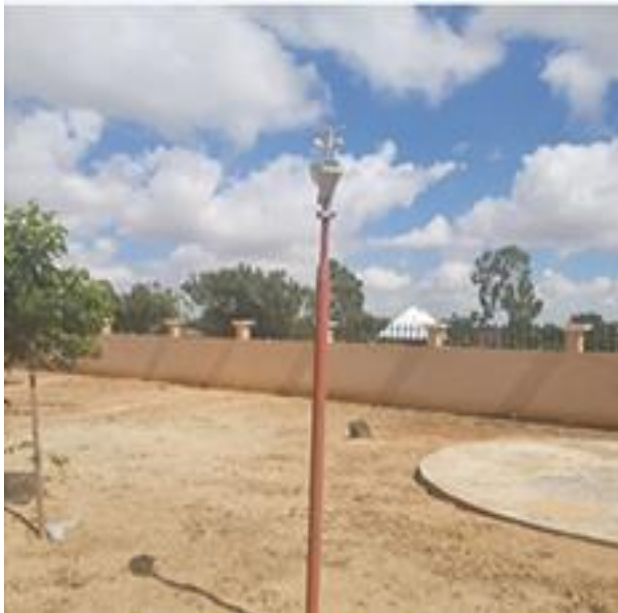
Outdoor sensor array installation (c)
