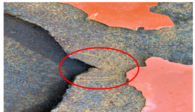
Figure 23 Cracks in the main fastening plate.
