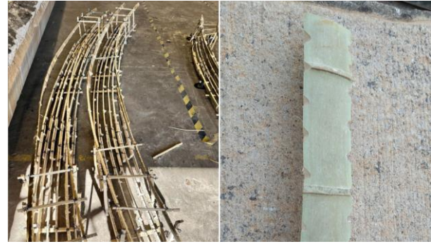
Figure 8: (left) Construction of bamboo cage; and (right) Notches in the bamboo pieces.
