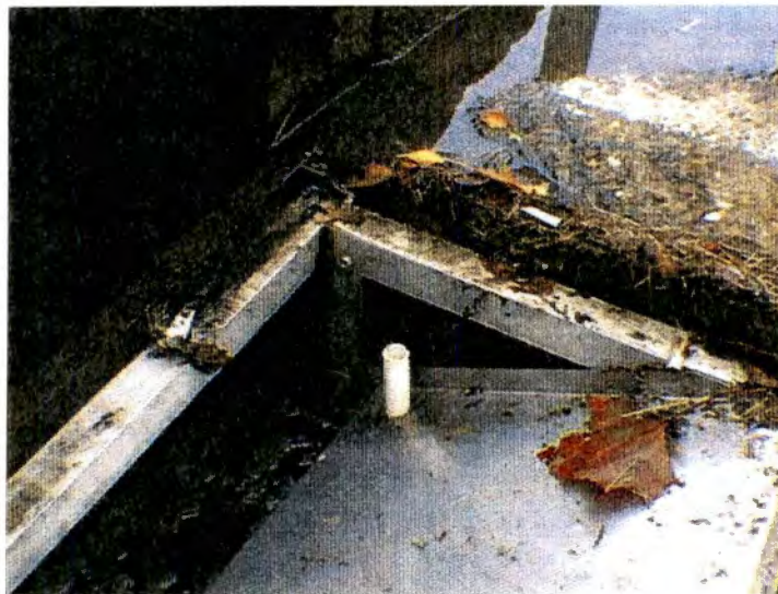
Figure 5-10. Low Flow Dripping Through Bypass (Site #2)
