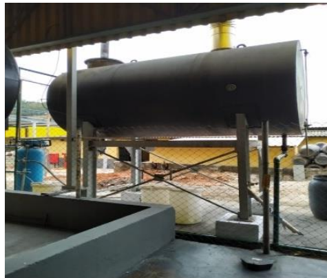
Figure 2 - Boiler water supply tank.
