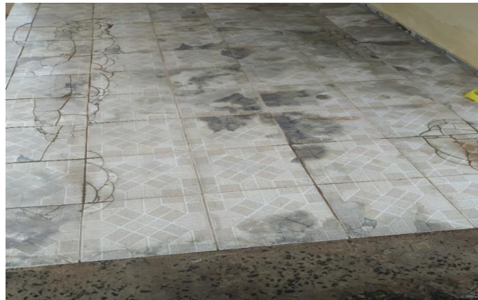
Figure 2 - Broken ceramic floor
