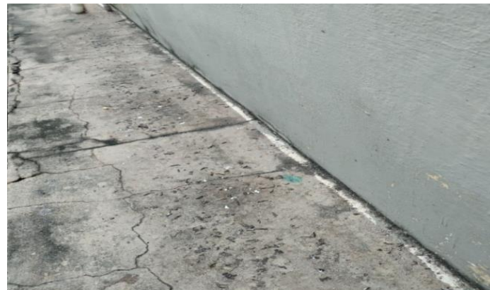
Figure 3 - Cracks in the sidewalk around the residence
