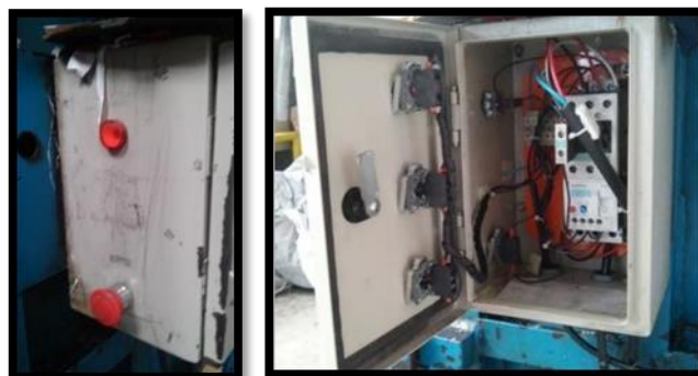
Figure 11 - Electrical panel and electrical controls Source: Author (2020)
