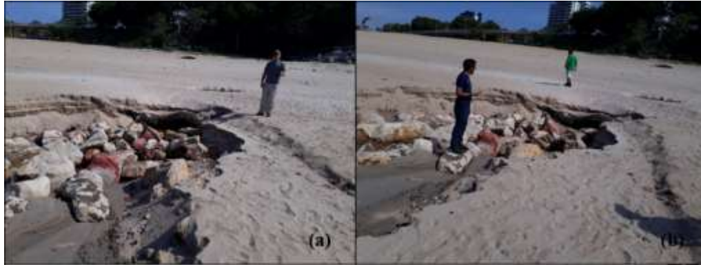
Figure 4: Features found on the transition surface of the embankment and natural beach, during the drought periods, in 2018 - a and b) Erosions with the appearance of the substrate rocks, approximately 2 meters wide, and 40 cm deep.
