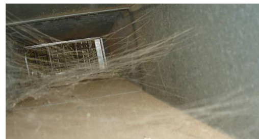
Figure 2. Insect presence housed in ducts.
