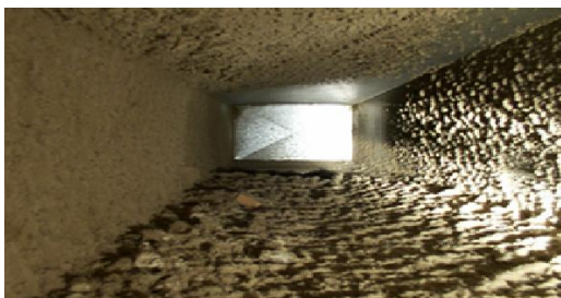
Figure 1. Ducts with dirt accumulation.
