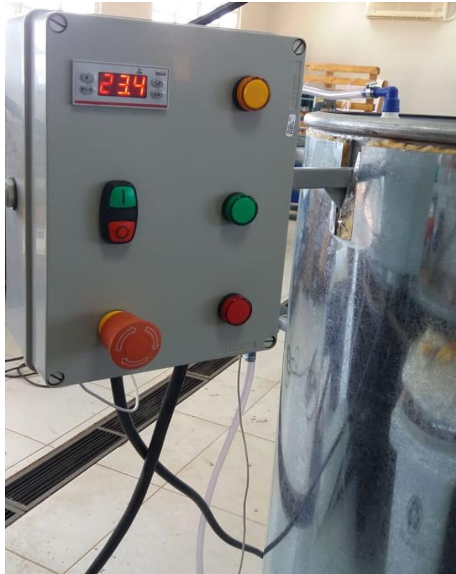
Figure 14. Reactor Electrical Panel Test.
