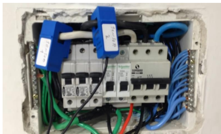
Figure 3. Integration of current sensors to the residential distribution board. SOURCE: Own author, 2019
