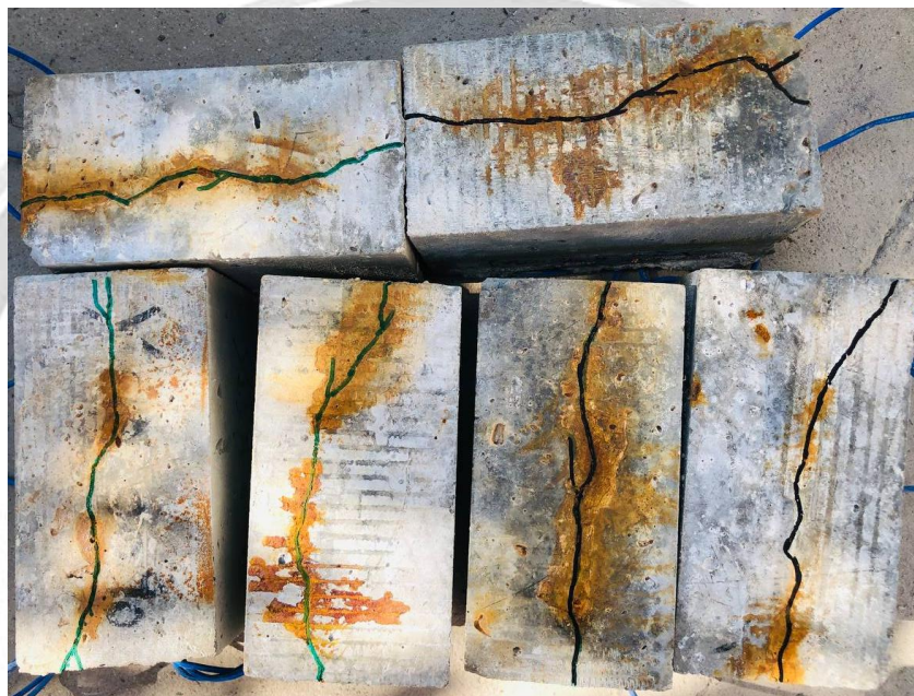
Figure 8: Crack Pattern for Concrete
