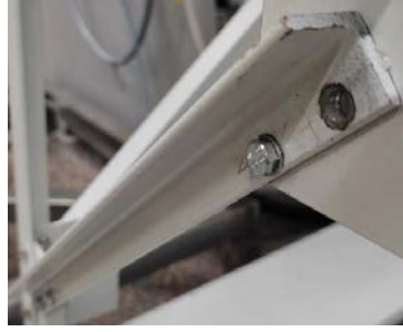
Figure 3: Damage type where the bolt is absent from the structure.
