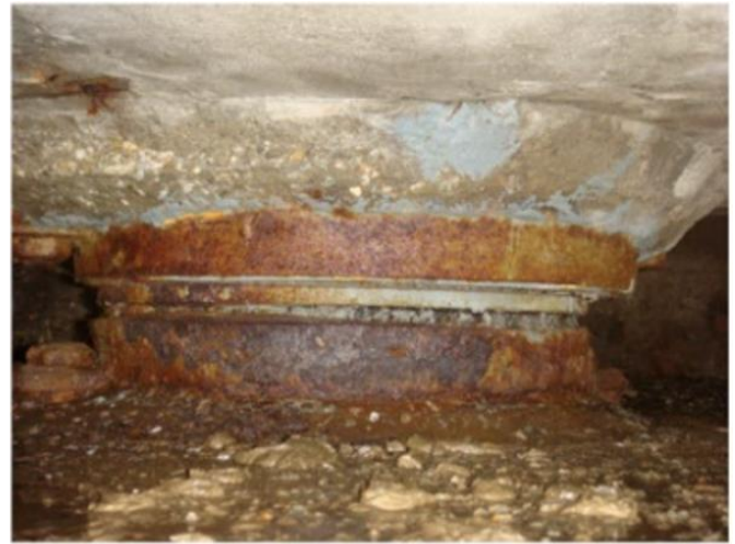
Figure 2 State of the bridge bearings before the start of the monitoring campaign.
