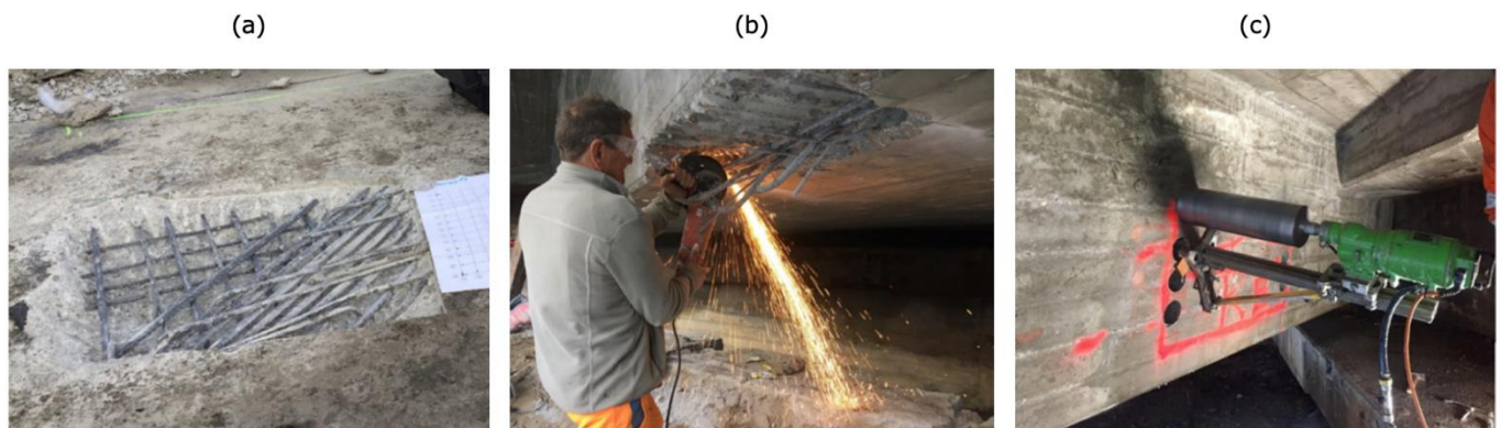
Figure 5 Example of the three damage patterns: rebar exposure (a), rebar cutting (b), and concrete drilling (c).
