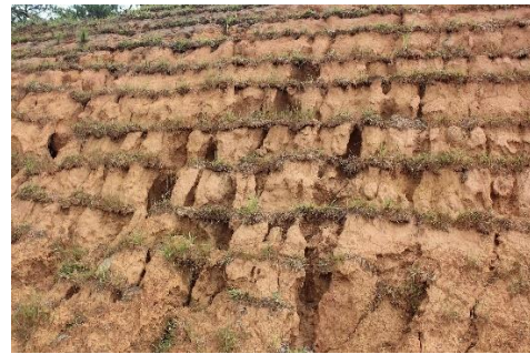
A slaking earthen road embankment
