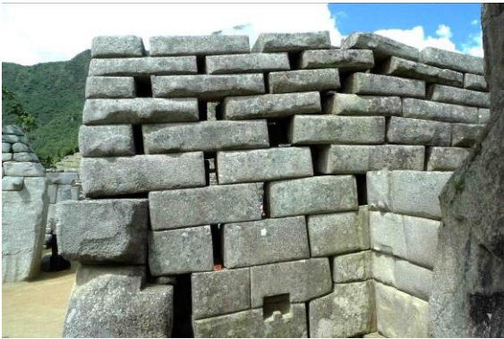
Figure 3: Displaced masonry blocks associated to creep movement in the Principal Temple.
