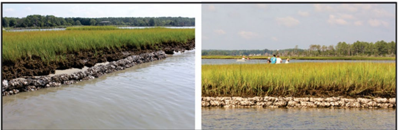
Figure 4-2. Construction of the 3-bag sill (left) and 6-bag sill (right) in August 2017. From Milligan et al. (2018). Photo credit: Linda Tjossem
