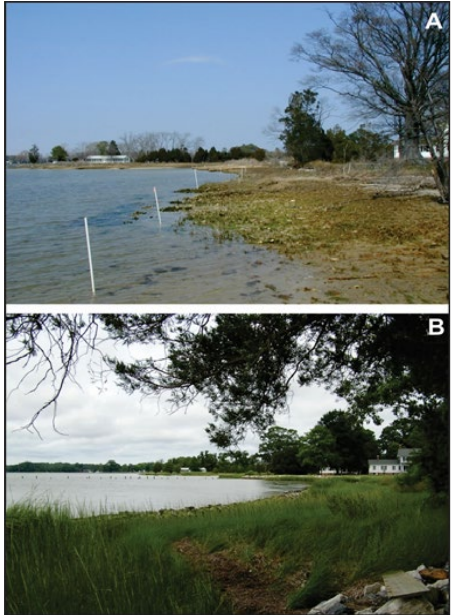
Figure 4-4. Hollerith marsh toe revetment/sill site A) before project with eroding fringing marsh in winter and B) after construction.
