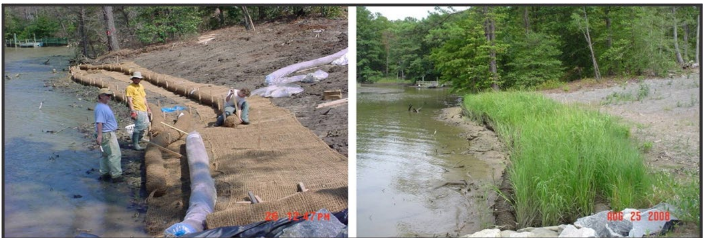
Figure 3-3. Coir logs and mats placed at toe of a graded bank for temporary stabilization while planted tidal marsh and riparian buffer become established. Photos by P. Menichino.
