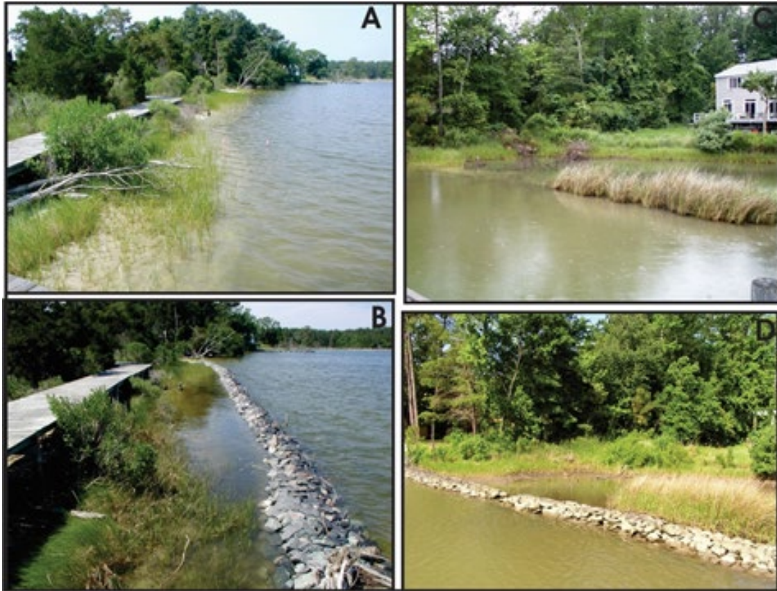
Figure 3-6. Photos showing marsh toe revetments A) before and B) after a project on Cranes Creek in Northumberland County and C) before and D) after a project on Mosquito Creek in Lancaster County, Virginia.
