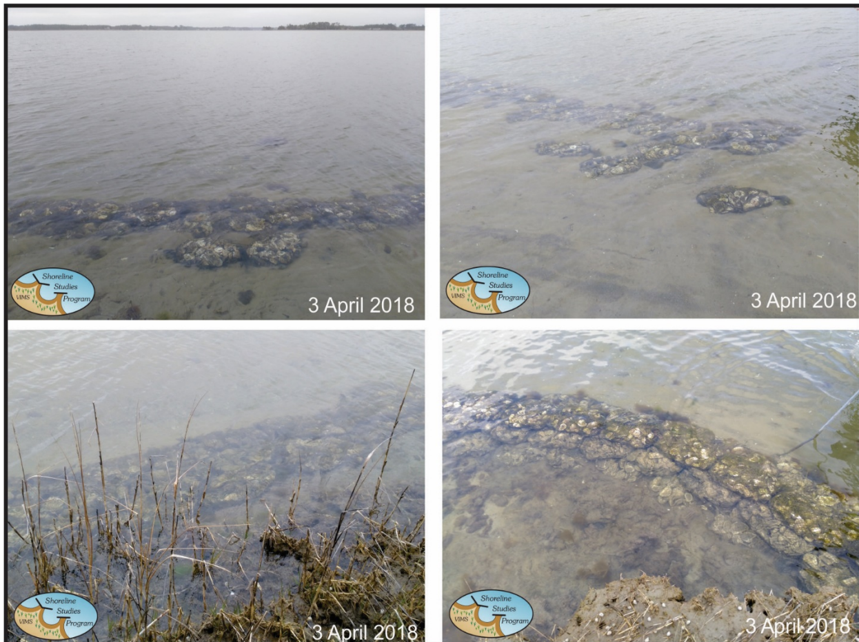
Figure 4-3. Captain Sinclair's Recreational Area oyster bag sill. The three-bag sill (top) that was placed on the southwest-facing shoreline has not been as stable. The top bag of some sections were rolled toward the shoreline. The six-bag sill (bottom) on the point and the southeast-facing shoreline has remained intact. From Milligan et al. (2018).
