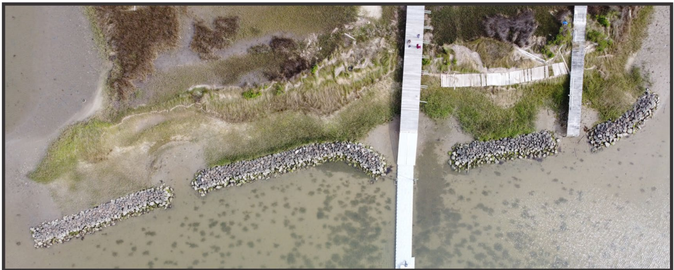
Figure 5-14. Drone imagery of the Captain Sinclair sills taken about 4 years after project installation (12 May 2020).
