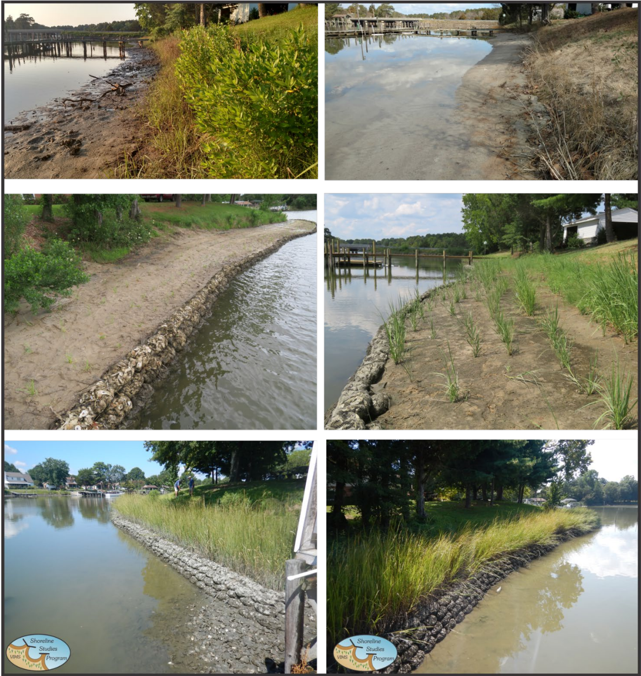
Figure 3-7. An example of the construction of oyster reef bags with sand fill and marsh grasses planted behind the structures. Top left: Shoreline prior to the project on 26 May 2016; Top right: after the sand fill was placed May 2017; Middle left: after bags were placed in May 2017; and Middle Right: after the grass was planted in July 2017. Photo credit: Walter Priest.
