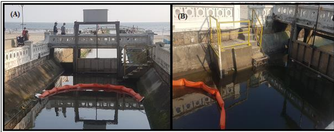
Figure - 10.6: Content barrier system (configured in "U" format), used to retain solid waste and other chemical and/or oily pollutants that are conducted into the urban drainage channels in Santos, Brazil.
