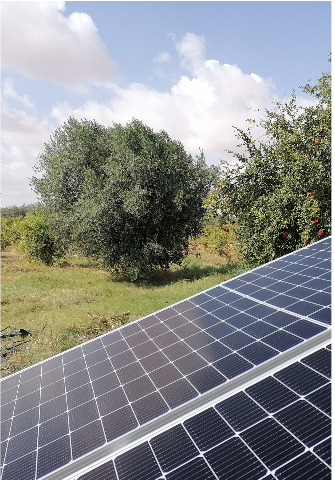
Solar panels at a farm in Chorbane, Mahdia, Tunisia, October 2021 (photo: Khaled Bedoui).
