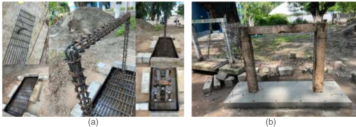
Figure 6. a) Centring work and b) casting of the reinforced concrete (RC) frames
