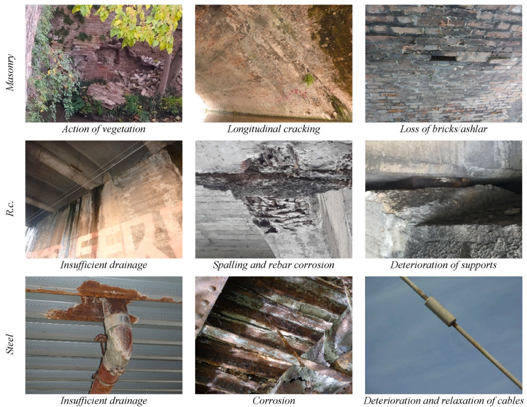
Fig. 23. Deterioration types commonly observed in bridges of Padova inventory.
