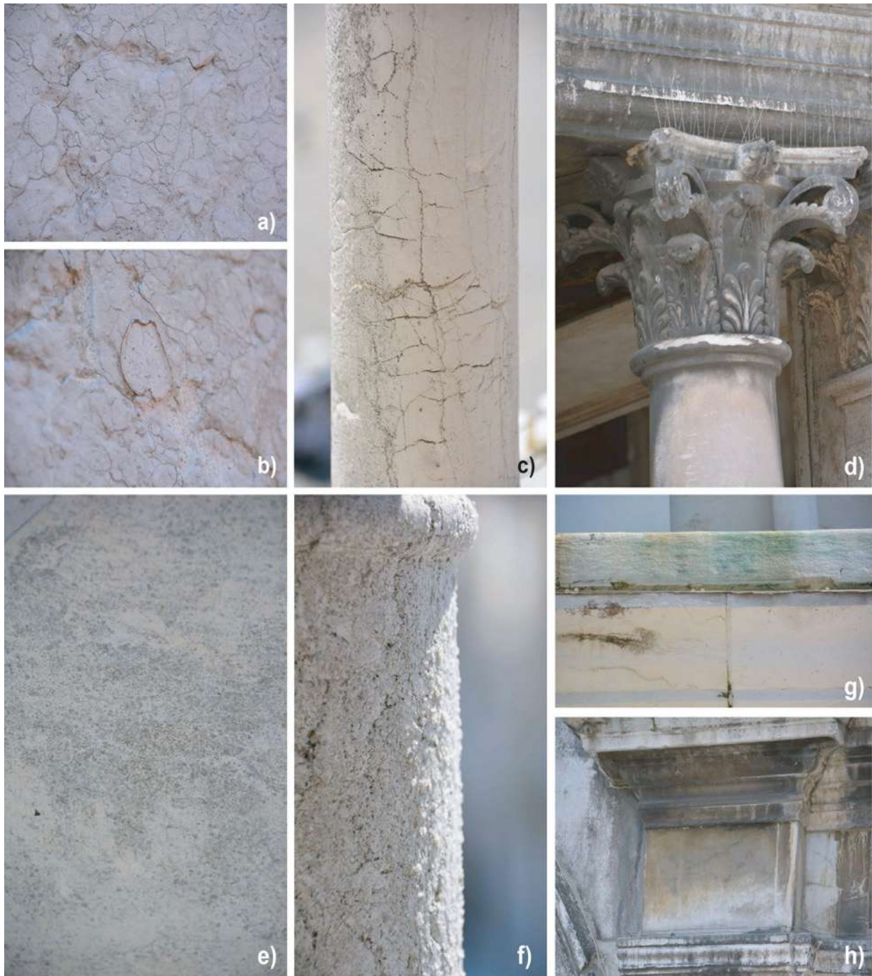
Fig. 6 Features induced by material loss: a, b differential erosion on Ammonitico Rosso from Verona slabs (eastern façade), c microkarst on Istrian Stone small columns (western façade). Discoloration and deposit: d black crusts on Istrian-stone Corinthian capitals (southern façade); e soiling on Scaglia Rossa slabs (western façade); f efflorescence on Istrian Stone small columns (western façade); g greenish staining on Istrian Stone (western façade); h yellowish patinas (southern façade)
