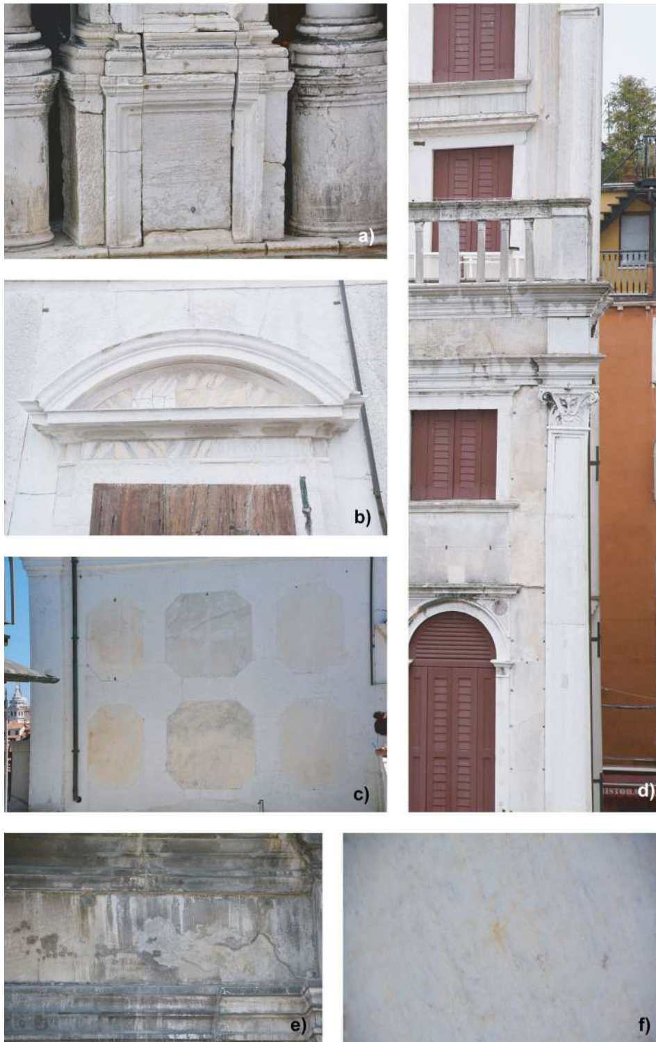
Fig. 4 Crack and deformation: a fractures on a pillar base (southern façade), and b on the marble slabs decorating the doorframe arch (eastern façade); c faint convex deformation on marble slabs (western façade); d lesene deformation (southern façade). Detachment: e blistering phenomena (southern façade); f sugaring phenomena on marble slabs (western façade)
