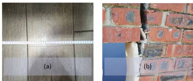
Figure 2. Structural damage resulting from the 6 February 2016 KwaZulu-Natal offshore earthquake (a) Long hairline crack at the Vodacom store, Hammarsdale mall, (b) Damage to a government subsidised Reconstruction and Development Programme (RDP) home in Hammarsdale.
