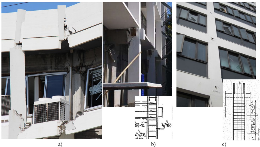
Fig. 1 Damage to reinforced beam–column joints: Uto City Hall collapse in the 2016 Kumamoto earthquake (courtesy of Jae-do Kang) (a); due to the 2011 Christchurch earthquake (Leon et al. 2012) (b, c)
