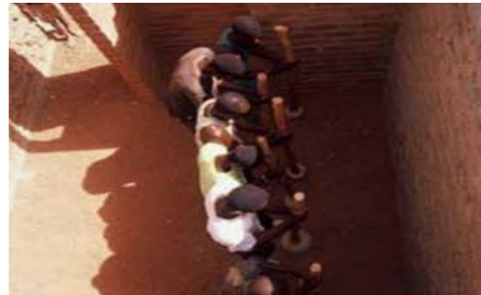
Figure 8 village men hand compacting the earth floor of the school (Galiano, L., 2018.)
