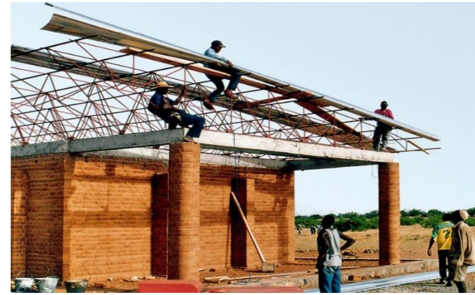
Figure 4 Construction of the Gando Primary School roof (Cano, E., Duchoud, S. and Ouwerkerk, E., 2022.)
