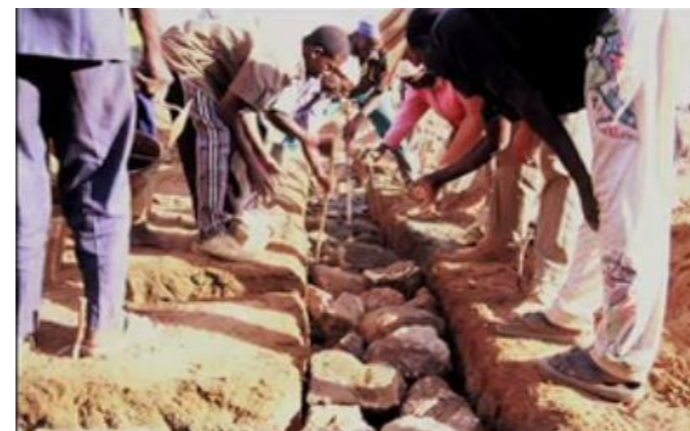
Figure 10 The foundation of the school is constructed from locally sourced stones (Galiano, L., 2018.)
